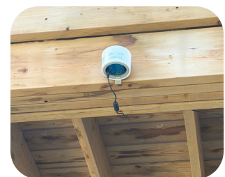
One of three air quality monitoring stations (band office) installed in Iskut.
